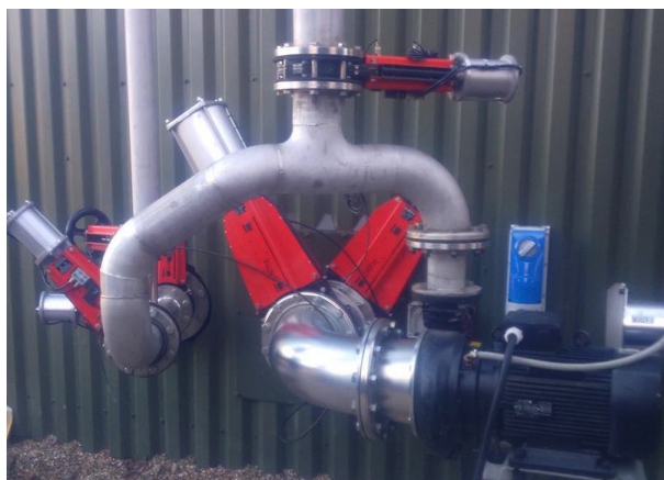
Landia's externally-mounted GasMix system at BIO Collectors' Surrey-based AD plant
