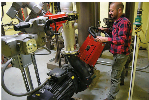
Tatulli verifies that the mixing pump suction valve is open.
