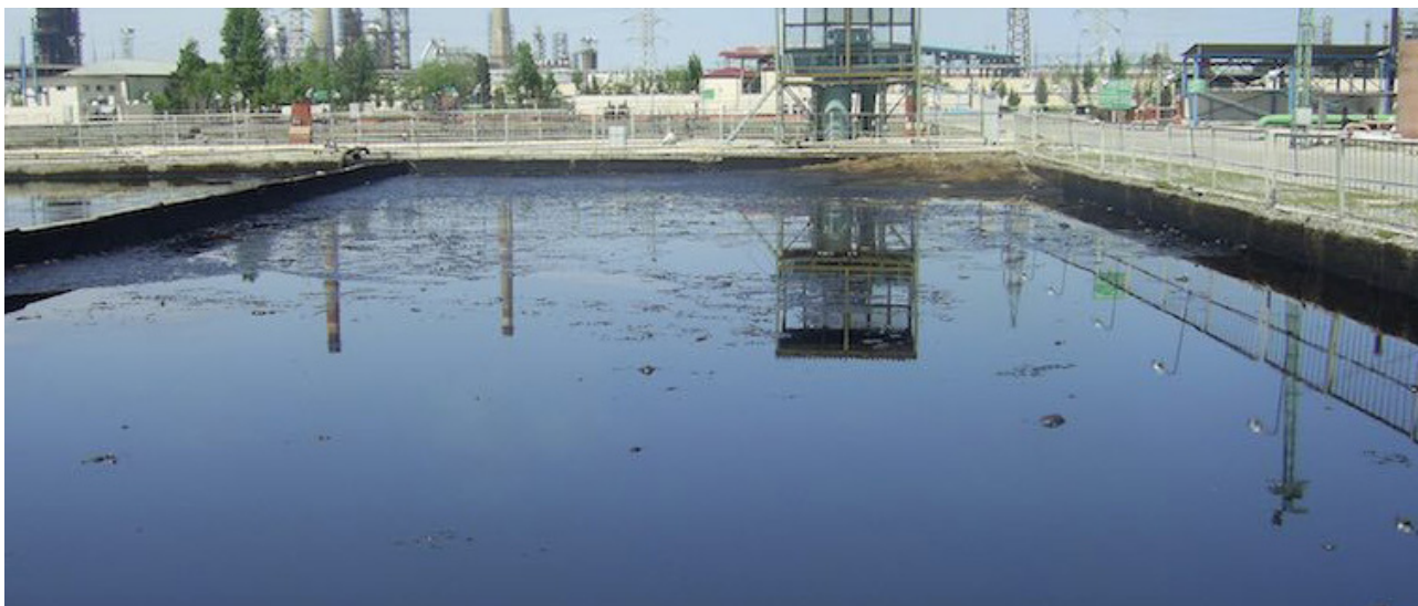
Open oil refinery lagoon in Azerbaijan, served by ultra-reliable Landia Chopper Pumps
