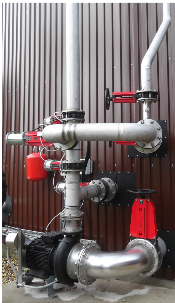
Externally mounted GasMix system
