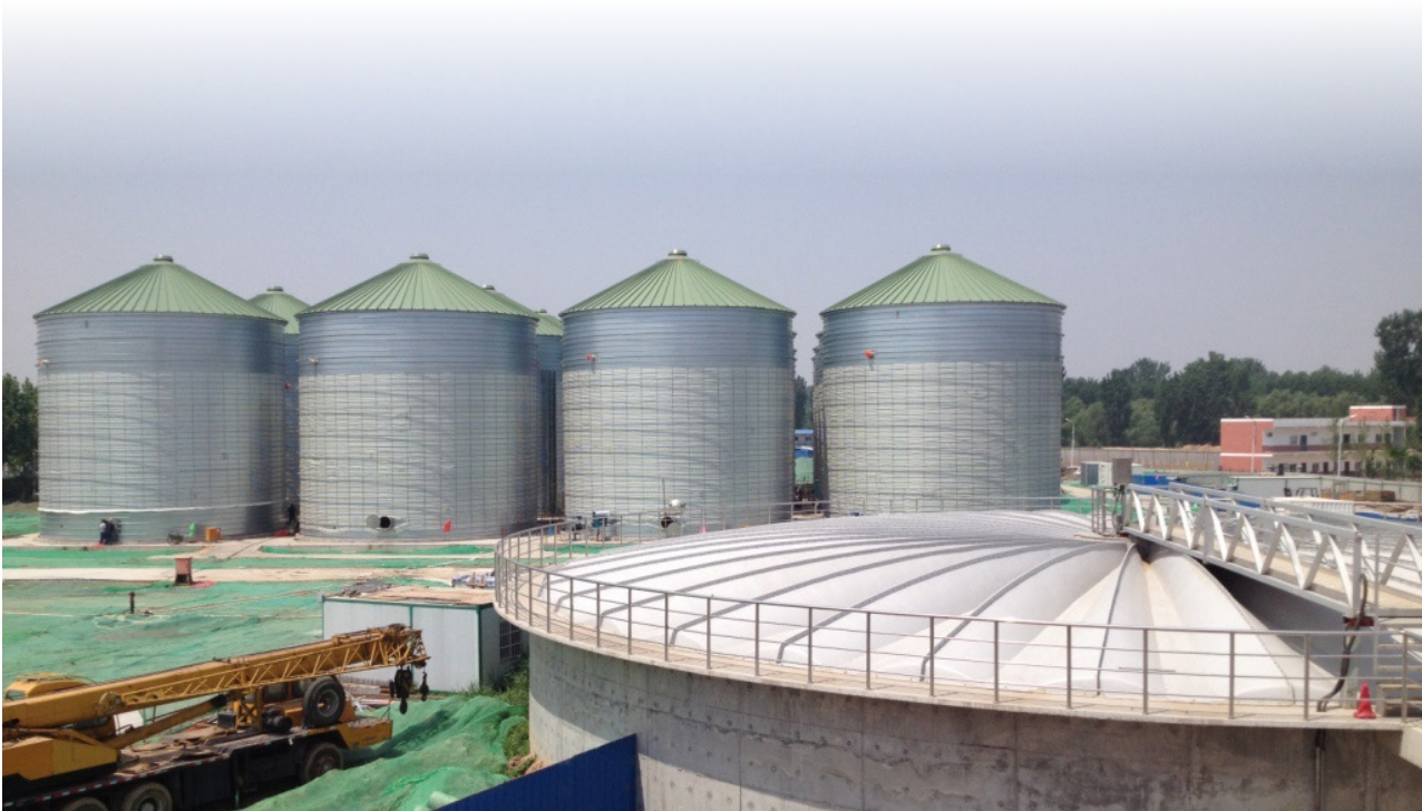
The new sludge handling facility in Matougang, China
