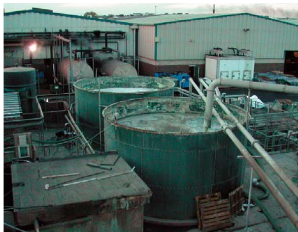
Dry-installed AirJet in tannery effluent aeration tank
