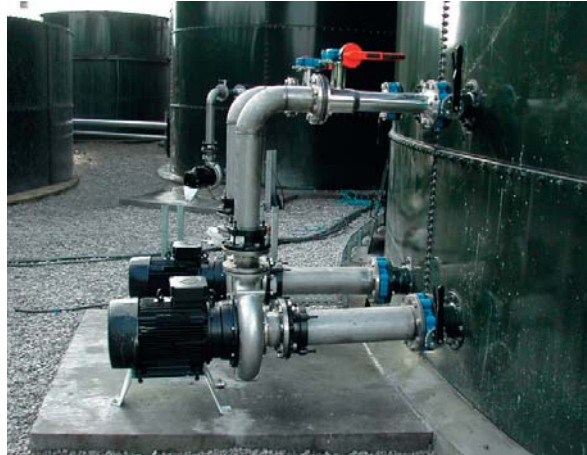
Dry-installed AirJets in jam factory effluent aeration tank
