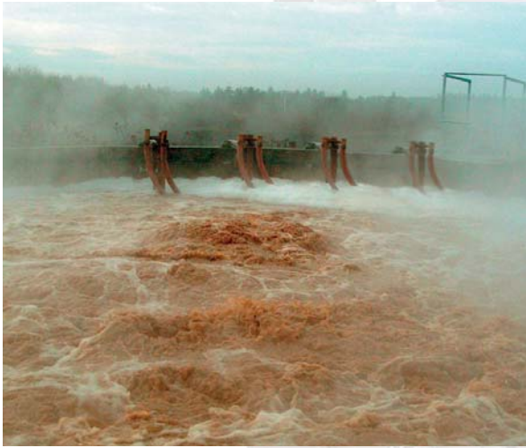
Submersible AirJets in paper industry effluent aeration tank
