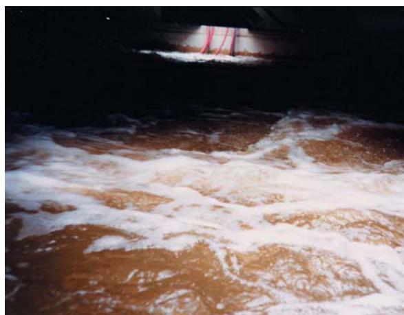
Submersible AirJets in leachate tank
