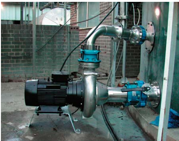
Dry-installed AirJet in tannery effluent aeration tank
