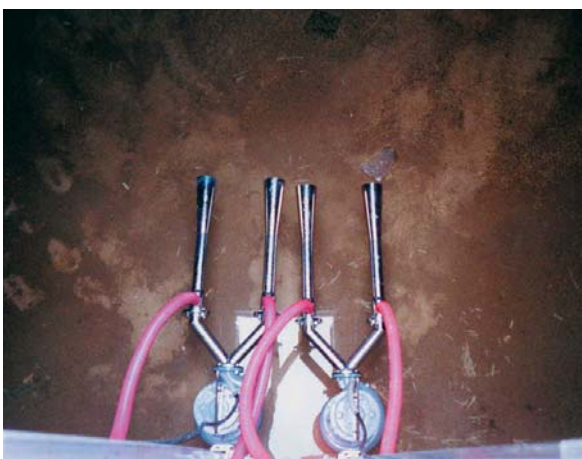
Submersible AirJets in leachate tank
