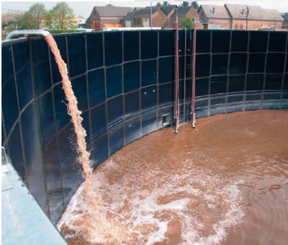
Submersible AirJet for odour alleviation in abattoir wastewater
